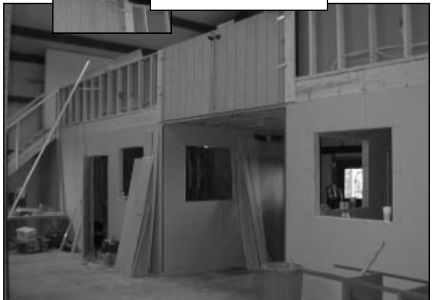
Below, the second floor of the warehouse under construction; inset, Bro. Larry Matson, contractor for the work
